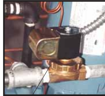
Typical water make-up solenoid valve
